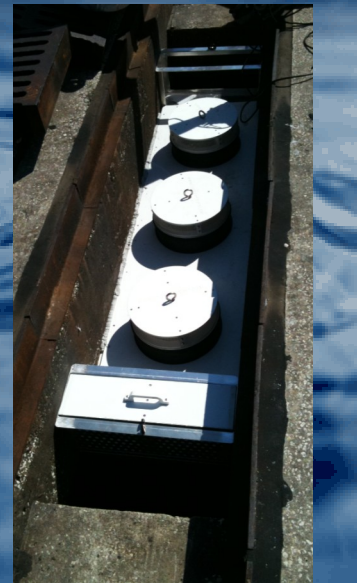
Hydrocarbon filters at airport (above)
